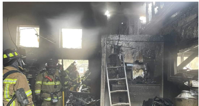
Significant damage to the outside and inside of an antiques store on Route 1 in Ogunquit. KENNEBUNK FIRE & RESCUE
